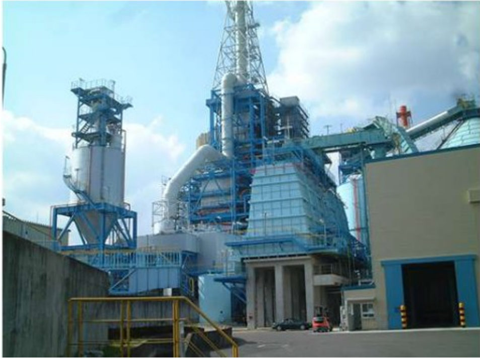
Fluidized Bed Boiler Batu Bara
